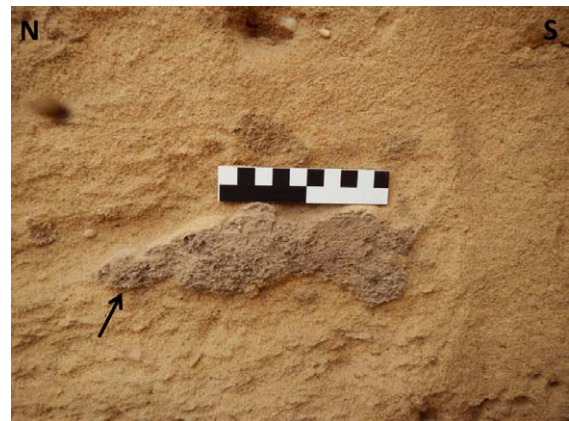
Fig. 95 Fragment of middle unit of exposure O-1. Visible fragment of mud brick with eroded surface (arrowed) – close-up from Fig. 89 (photo J. Trzciński)
